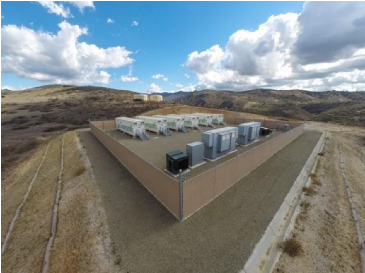
2MW/6MWh battery storage system installed by Greensmith for a privately owned utility in San Juan Capistrano, near Orange County, California - to provide peaking power and defer grid investment SUPPLIED PHOTO
