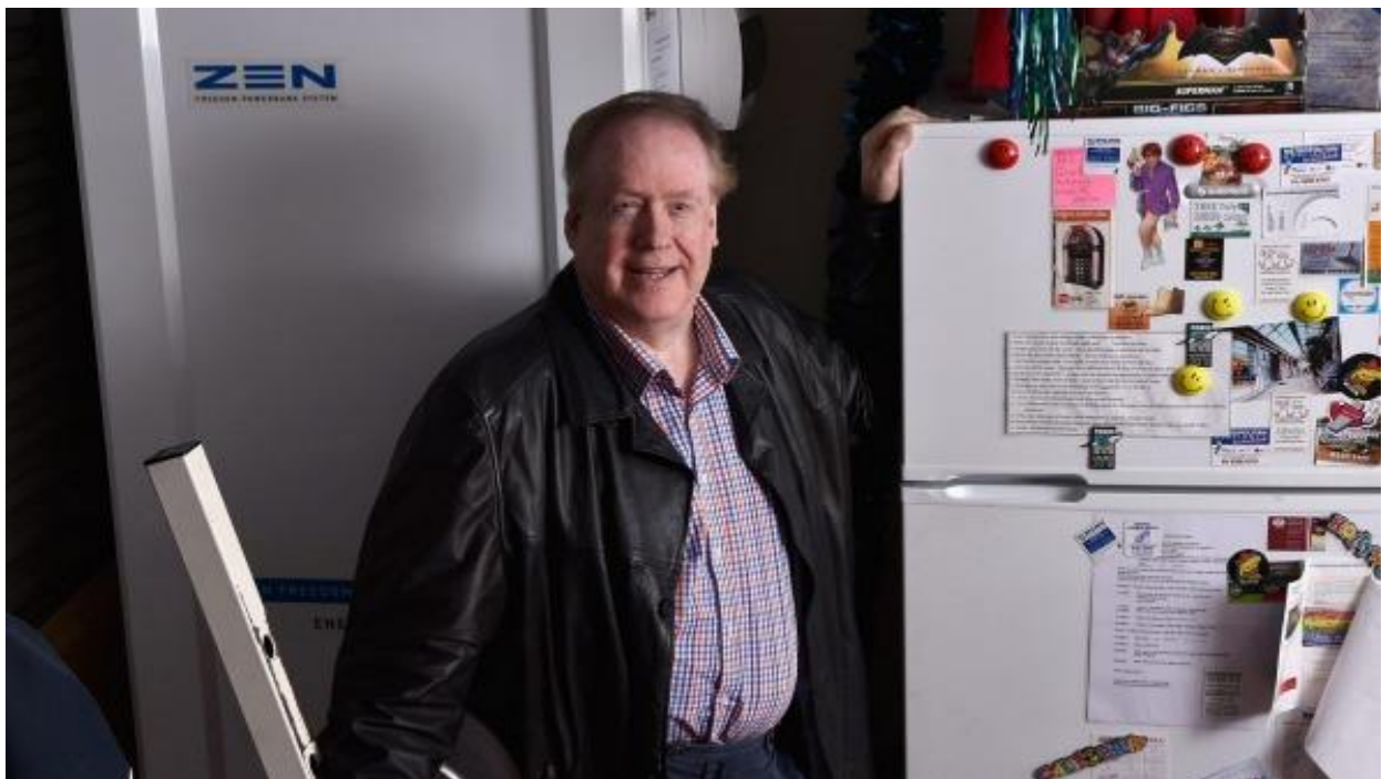
Adelaide radio host Leon Byner with his 20KWh home battery system installed by ZEN Energy. The company says batteries are ready for large scale deployment to shore up the power grid. David Mariuz
