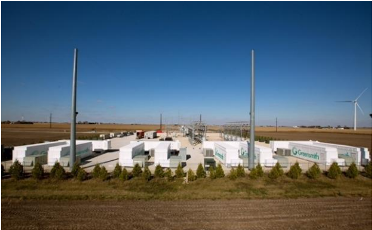
18MW/9MWh battery storage system installed by Greensmith for transmission company PJM to stabilise the grid in rural Illinois. Eddie Hackelton
