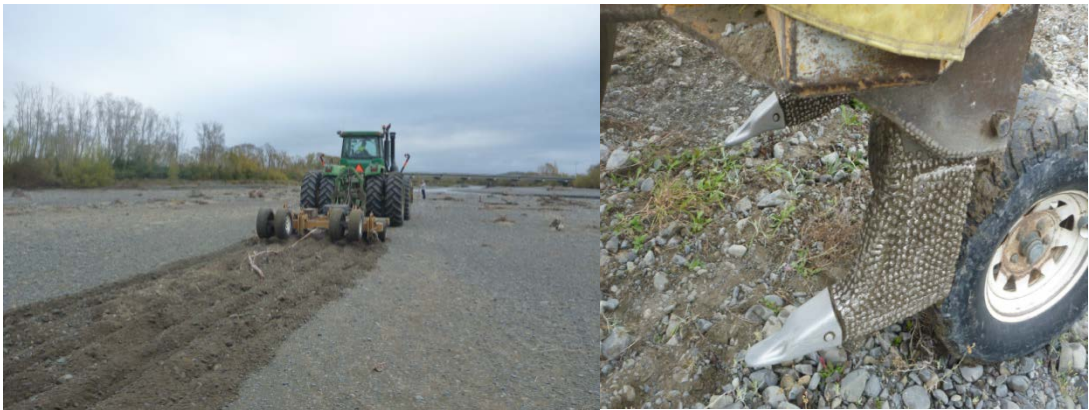
Figure 1 Tractor and trailer unit raking a beach on the Waipawa River in the Hawkes Bay (left); The 'ripping blades' used to break the armour layer (right).
